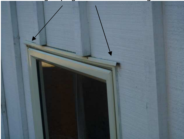
Head flashing sloping back due to cladding
