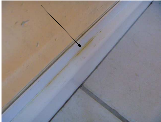
Leak from shower screen
